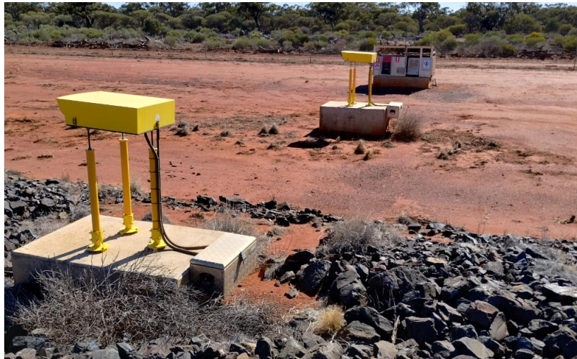
Figure 4: Existing PAPI lights
