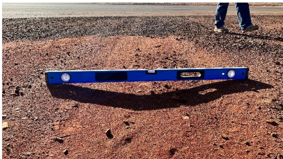
Figure 5: Water Erosion Damage in places
