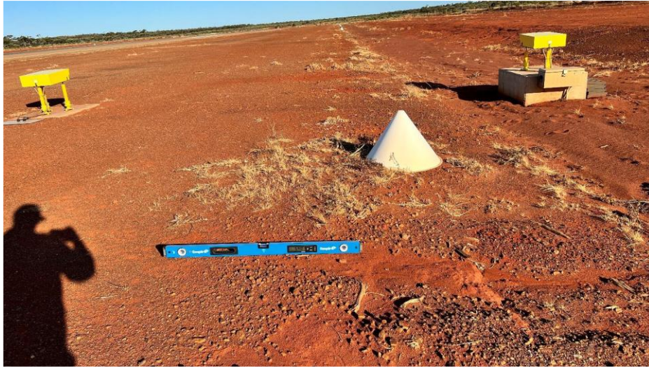
Figure 6: Graded strip next to runway exceeding permissible downward slope
